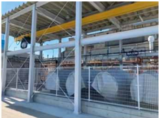
Storage tank for ammonia fuel
