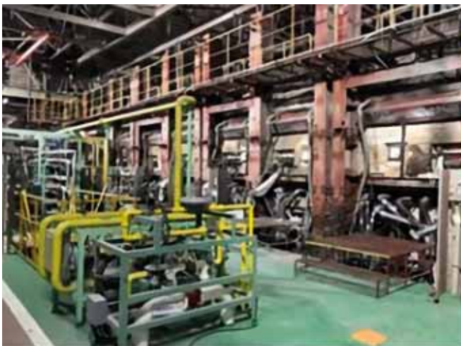
Glass melting furnace in which this demonstration test was conducted
