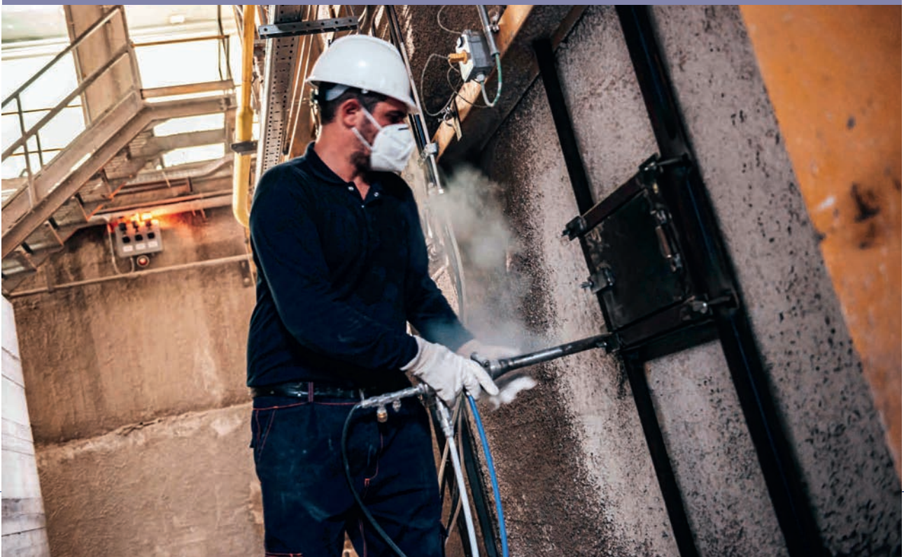
Pic.1 - The installation of Stara Glass SNCR systems is performed while the furnace is running
