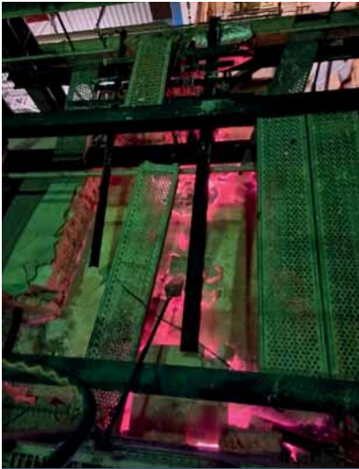
Fig 7. Damaged furnace crown
