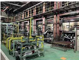
Glass melting furnace in which this demonstration test was conducted
