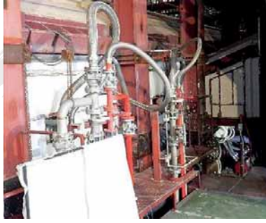
Glass melting furnace in which the demonstration test was conducted
